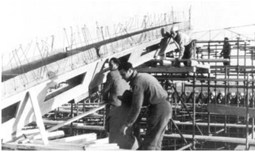
Figure 10 Sports Palace: placement of a V-shaped element for the dome (Nervi 1965a)
