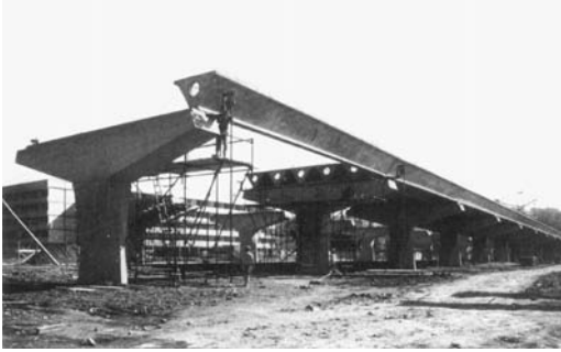
Figure 12 The Corso Francia Viaduct: the positioning of a beam on a support (Nervi 1965b)
